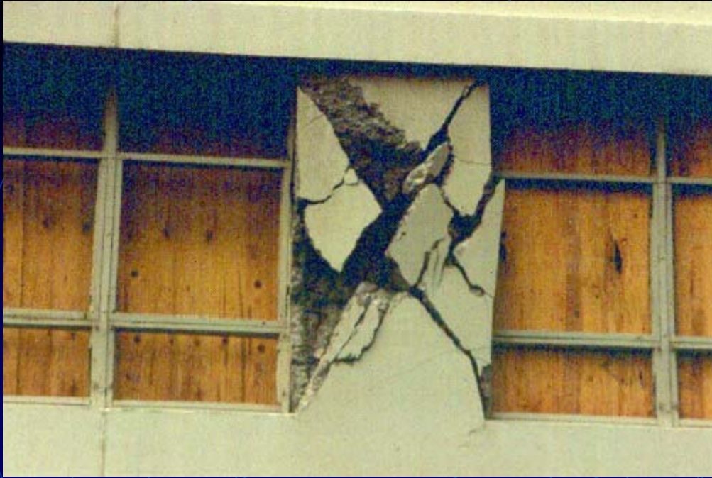
Short column mechanism, Northridge, 1994
