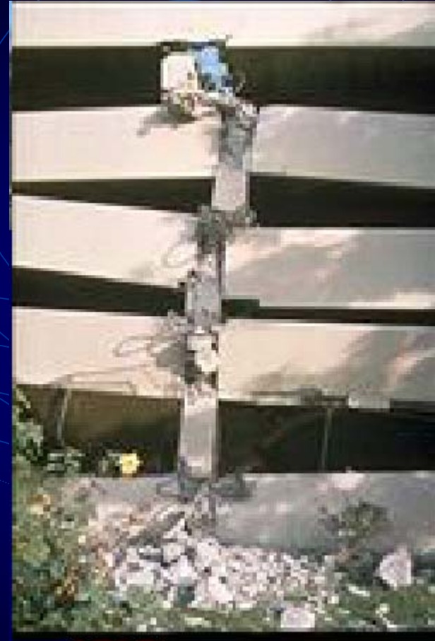
Vulnerability of structural system, Northridge, 1994
