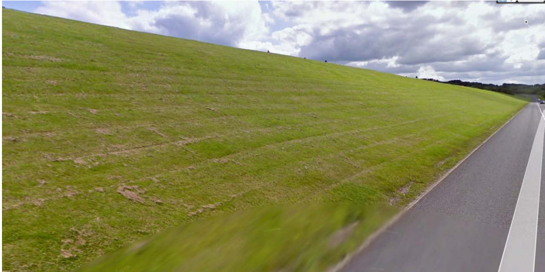
Figure (5). Downstream view of the reconstructed Earth Embankment of the Carsington Dam.
