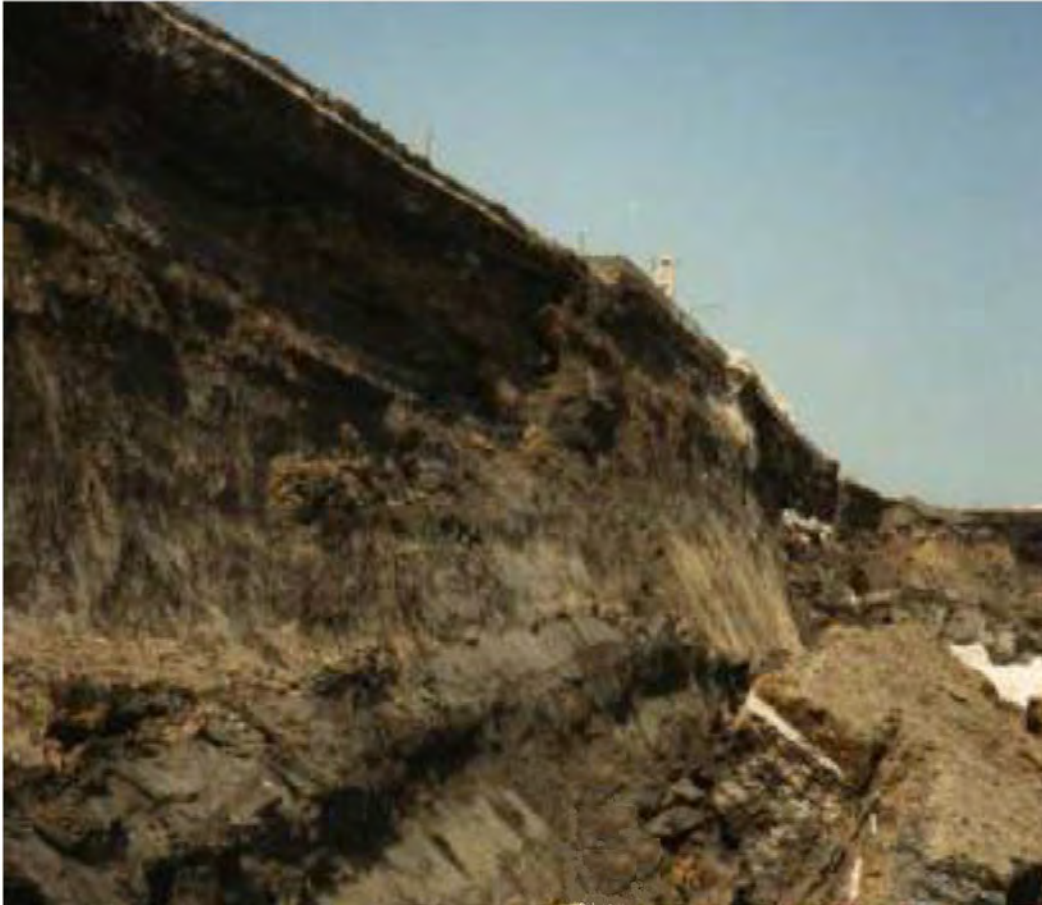
Figure (4). Close up of the upstream slip failure surface of the Carsington earth embankment dam, showing the slip propagated along the embankment with an embankment crest slumping of 11 m (Environment Agency, 2011).
